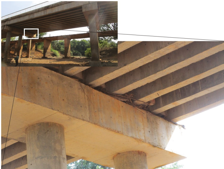
Figure 16. Pieces of branches blocked under the bridge deck of the new bridge of Komba on the Komba River (Upper Koliba/Corubal basin) after the flood of 2018. On the small picture: the new (2012) and, in the back, the ancient bridge (1950s).
